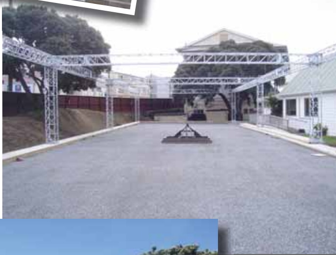
Above: Supports for the practice nets in place, the finishing touches are made to the subgrade
